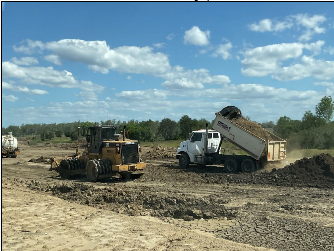
Picture 2: View of the Filling Operations
