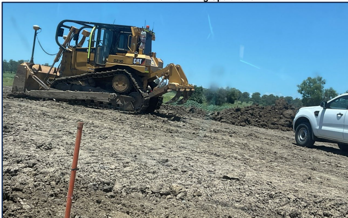
Picture 2: View of the Filling Operations
